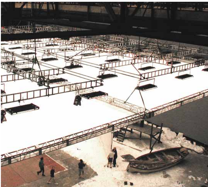
Flathead 80 and Image 85 fixtures, as space lights on made-for-TV movie stage
